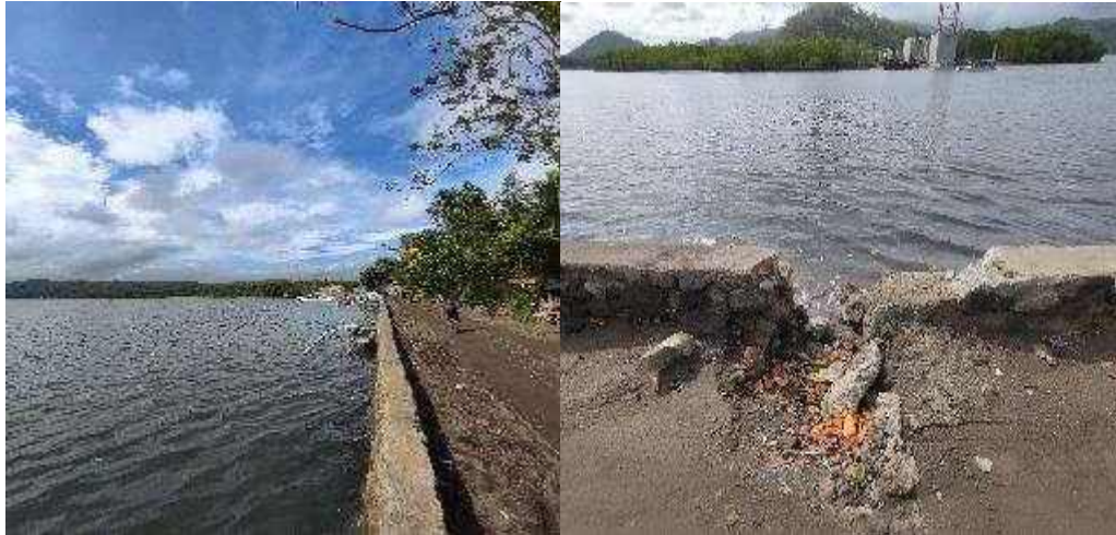
Figure 7 Existing condition of embankments in South Lembar village
